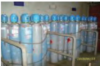
Special Gas Cylinder Warehousing
