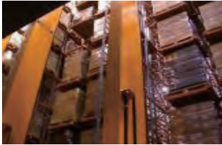
Automated Storage / Retrieval System
